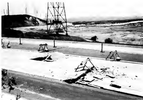
Photo 13. Compressional breaks in southeast-bound lanes of Golden State Freeway bypass, approximately at contact between fill to right and cut in Saugus Formation to left. View south also shows slide mass of Lower San Fernando Dam in now-empty reservoir in right background. Small landslides formed in hill in left background, and rocks fell from bore cut during the shaking.
